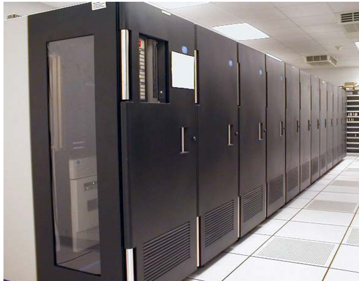
Automated Tape Library (ATL) IBM 3494
